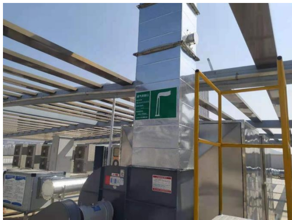
废气排放口标牌
