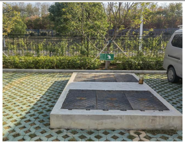
污水排放口标牌
